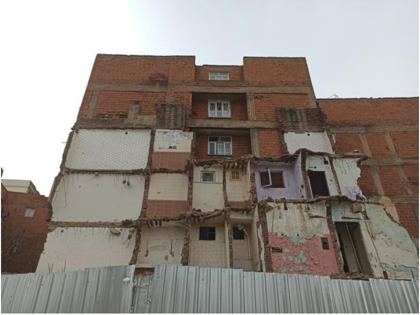
Picture 6. Half building , at one of the passage points from emptied Sur to old Sur 33
